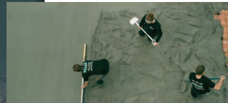
Project with University of South Australia - pouring of reinforced Crumb Rubber Concrete (CRC) for use in Australia’s residential construction industry.
